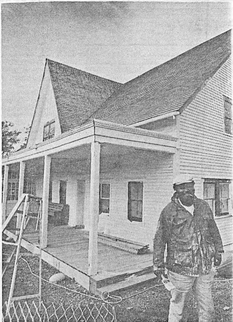
The Erskine House, a.k.a. the Baranof Museum, gets a new coat of paint. Buford Jackson, left, and Don Foster of Ideal Painting and Decorating.
