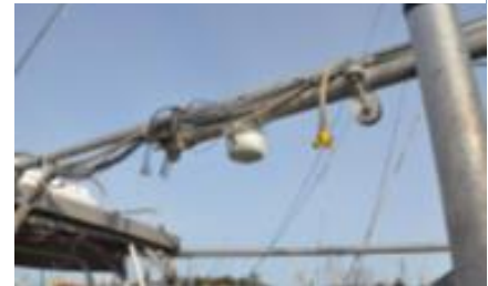
Figure 2 Typical placement of deck camera
