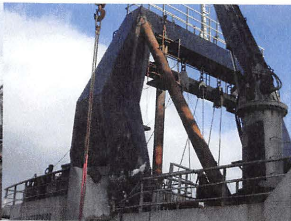
Damage to the gantry of F/V Kodiak Enterprise
