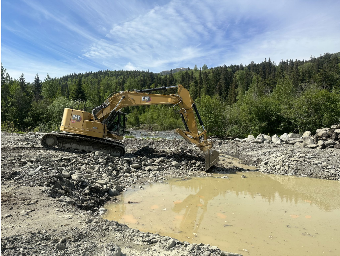
Figure 2. Rewatering a side channel of Resurrection Creek following restoration of the previous mine site. Photo Credit NOAA.
