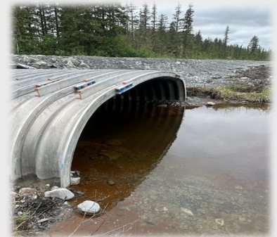
Completed fish passage culvert replacement on the Cordova Highway in Cordova, AK.
