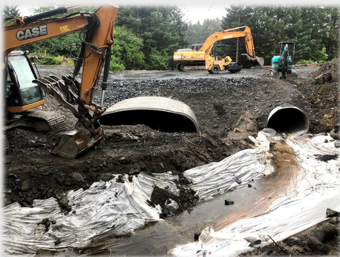
Fish passage restoration project under construction on the Buskin River in Kodiak, AK.
